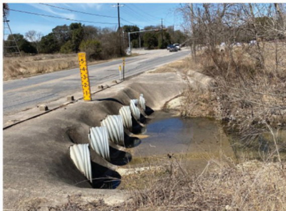
Conditions of low water crossing at Menger Creek and Old San Antonio Road.
