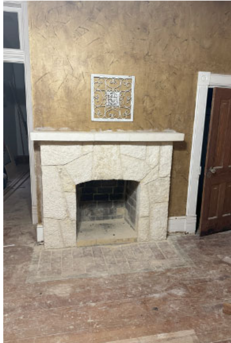
Existing fireplace in parlor, existing wood floor uncovered from 4 layers of material including concrete.
