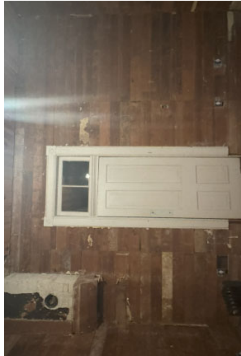
Typical existing door and transom, with old cook stove chimney still in place.
