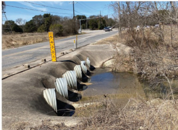
Conditions of low water crossing at Menger Creek and Old San Antonio Road.
