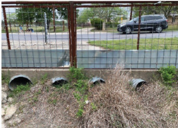
Conditions of low water crossing at Unnamed Tributary A Creek and Adler Road.
